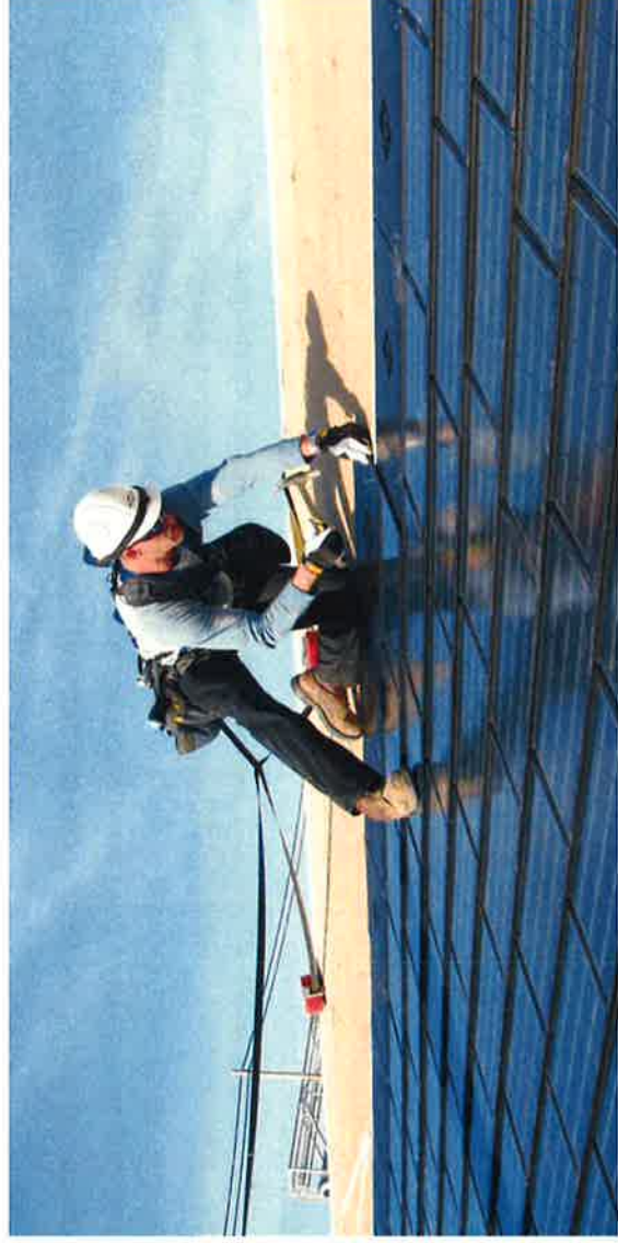
Integrated solar roof panels
